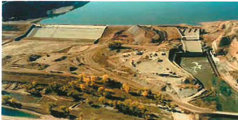
Emergency spillway made of RCC on the dam wall to prevent overtopping
