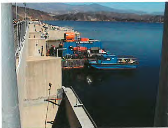
Divers boat and barge at spillway. Cofferdam used on spillway in foreground.
