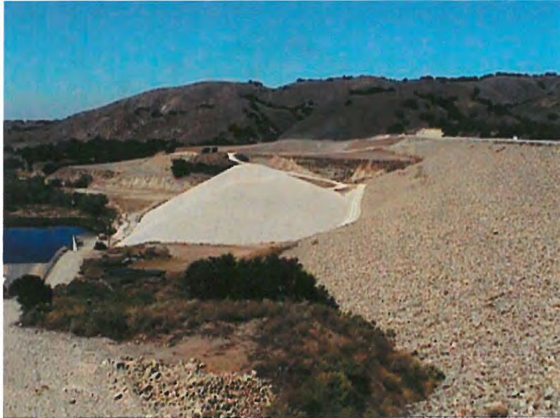
The white material is a berm that is designed to stop the dam wall on the right slipping down stream.
