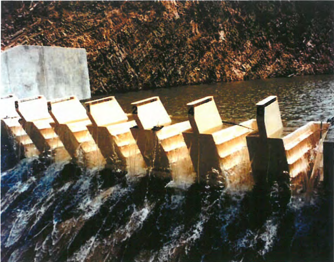
Fusegate spillway using the labyrinth design to increase the water flow.
